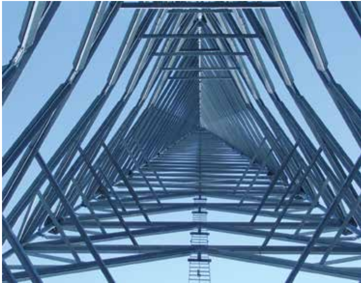
Looking up a Rescue 21 radio tower in Cape May, New Jersey.
